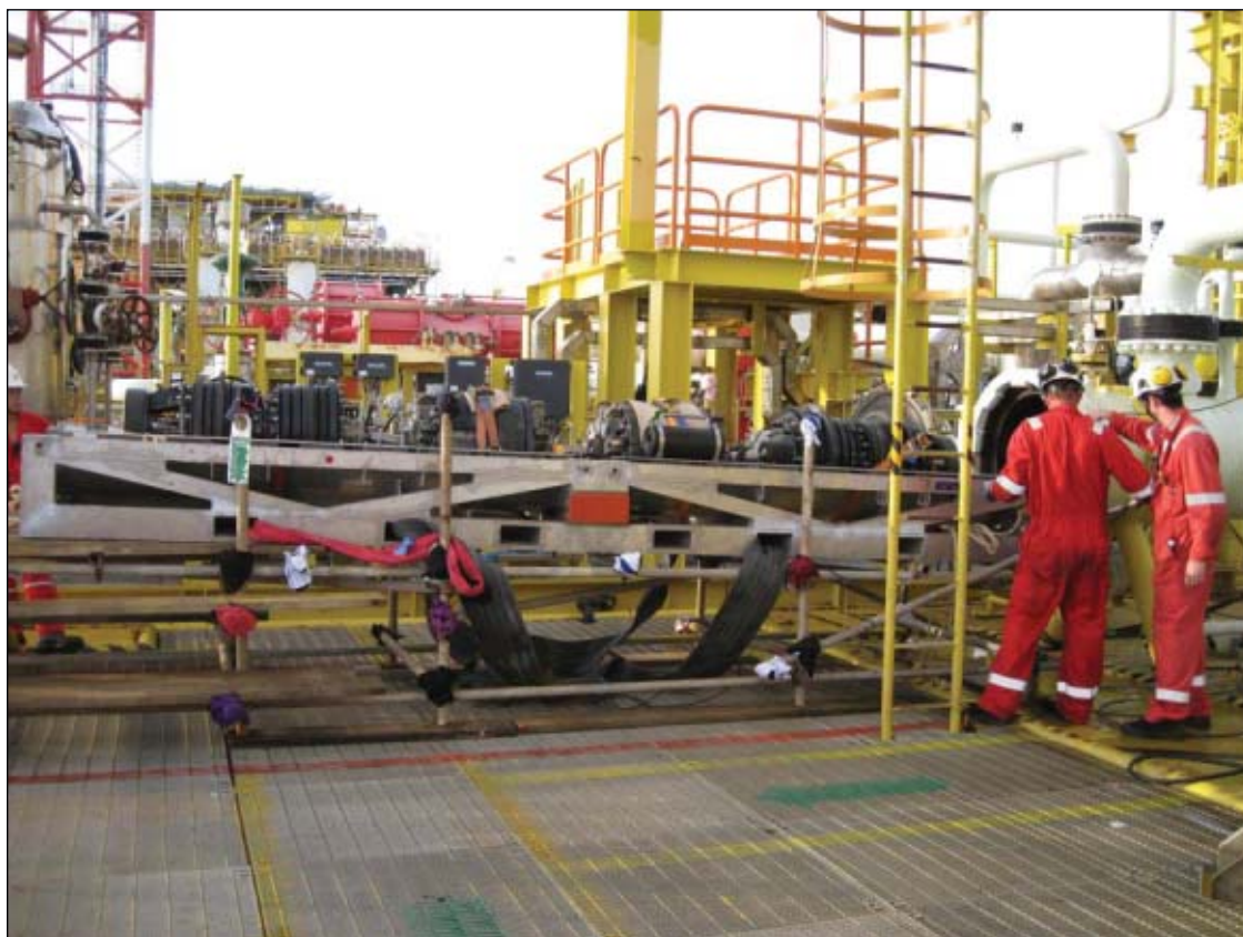
A team prepares to load the pressure isolation tool into a pig launcher as part of valve replacement at Sarawak Shell Berhad's M3 platform offshore Malaysia (Source: TDW Offshore Services AS; Fig. 2).
